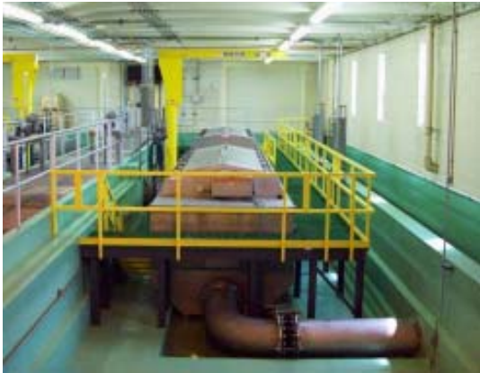
FRP Platform and Handrail installed above water treatment tank.
